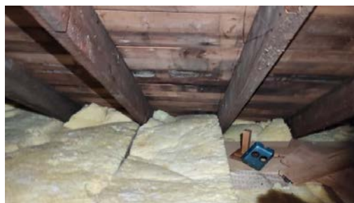
Manglende lufting i raft.
