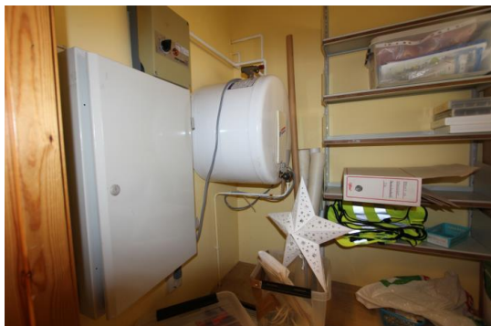
Veggmontert vvs tank.
