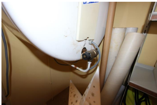
Veggmontert vvs tank.
