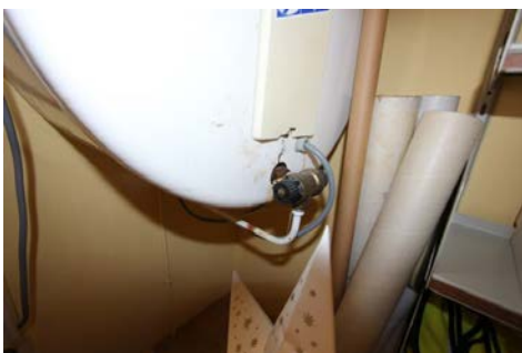
Veggmontert vvs tank.
