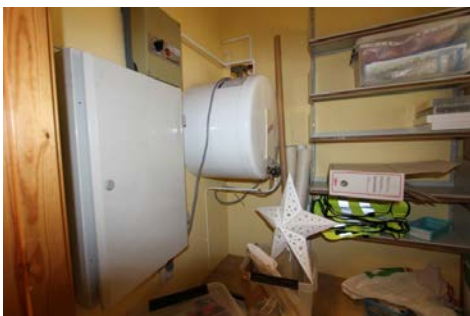
Veggmontert vvs tank.
