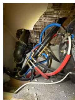
Rør stamme i himling over bad.
