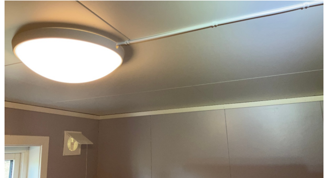
Himlingsplater i himling
