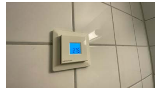
Termostatbryter for varmekabler.
