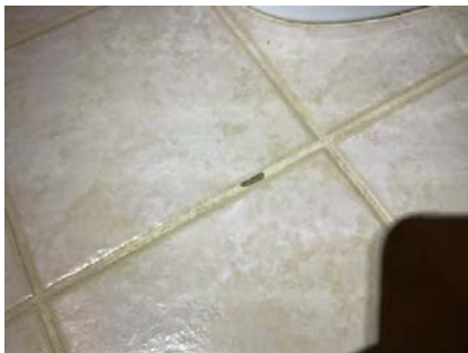
Hull i fuge.
