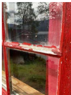
Manglende tetting mot glass inn mot stue.
