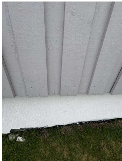
Sprekker i panel.
