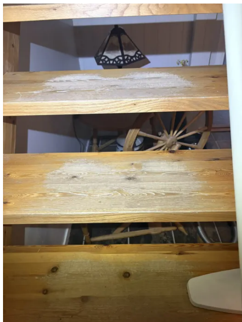
Overflate i trapp.
