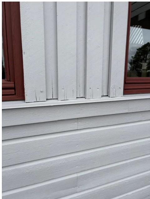
Sprekker i panel.
