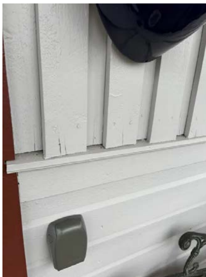
Sprekker i panel.
