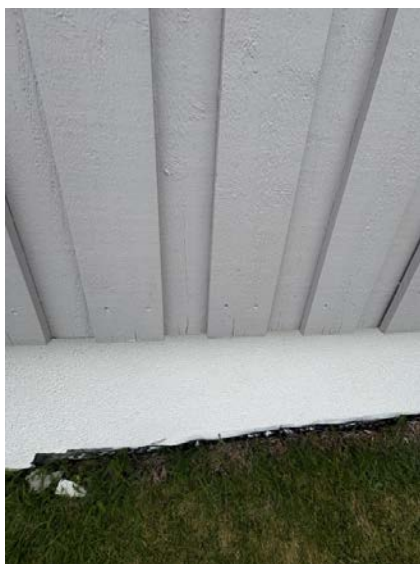
Sprekker i panel.
