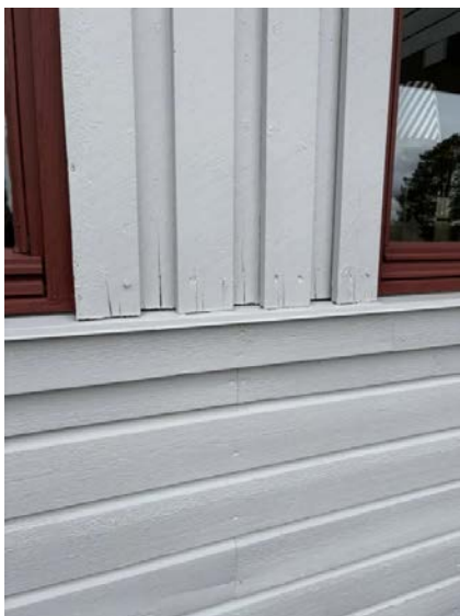
Sprekker i panel.
