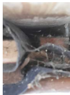
Manglende musesperre under kledning.
