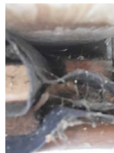
Manglende musesperre under kledning.
