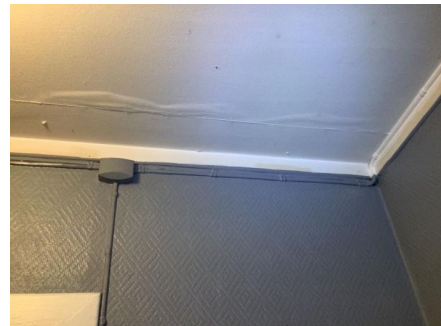
Folieslipp i himling.
