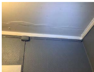
Folieslipp i himling.
