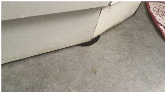
Sluk under servant.
