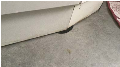
Sluk under servant.
