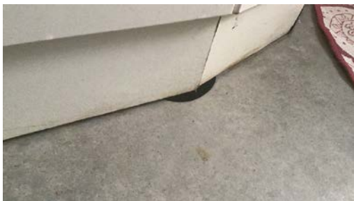
Sluk under servant.
