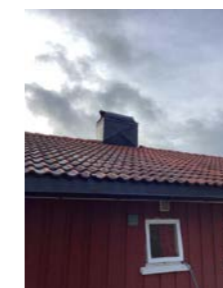
Manglende adkomst for feier.
