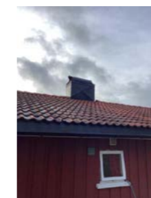
Manglende adkomst for feier.
