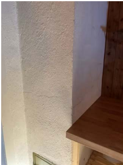
Sprekker i pipe.
