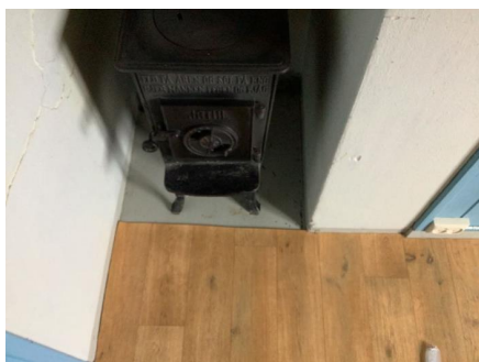
Manglende ildfast plate foran ildsted.
