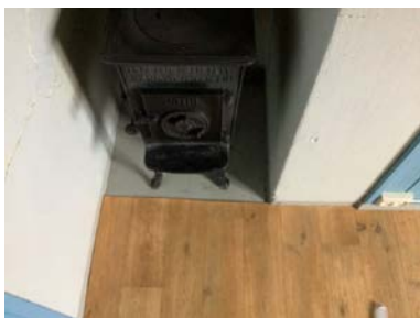
Manglende ildfast plate foran ildsted.
