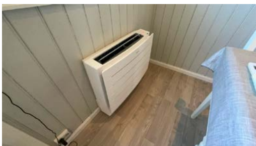
Varmepumpe, innvendig aggregat.
