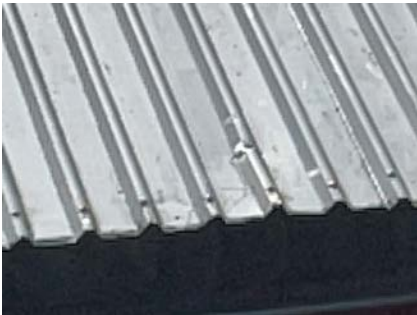
Noe bulker i takplater.
