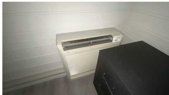
Varmepumpe, innvendig aggregat.
