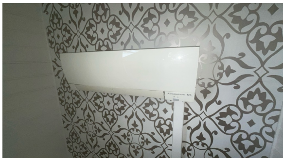
Varmepumpe, innvendig aggregat.
