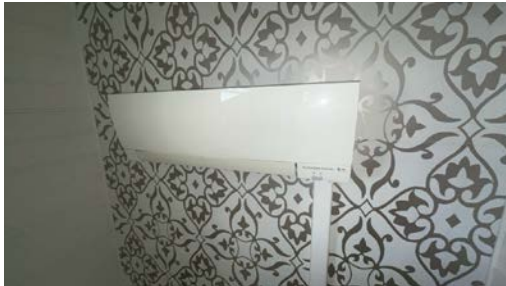
Varmepumpe, innvendig aggregat.
