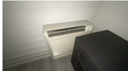
Varmepumpe, innvendig aggregat.
