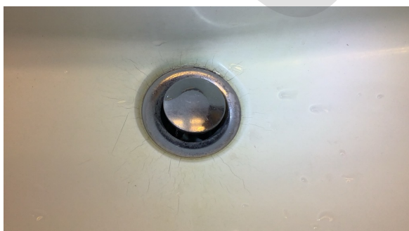
Riss i servant.
