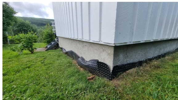
Grunnmursplast mangler klemlist.
