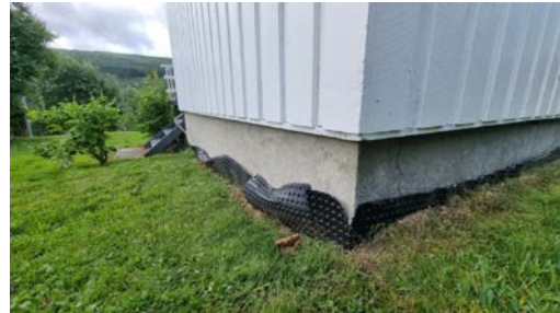
Grunnmursplast mangler klemlist.
