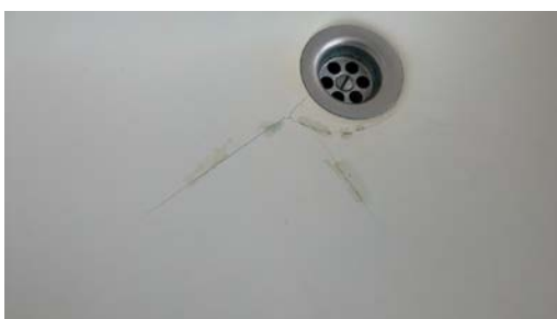
Krakelering i servant.
