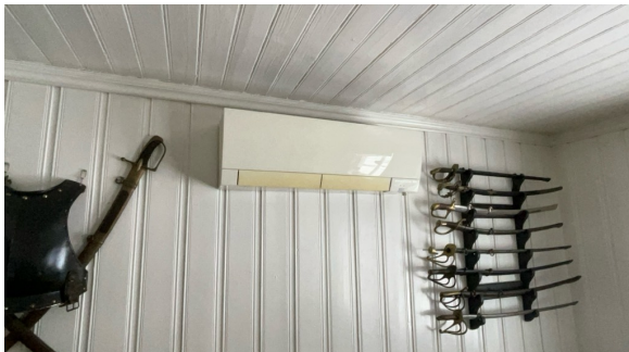
Varmepumpe, innvendig aggregat.
