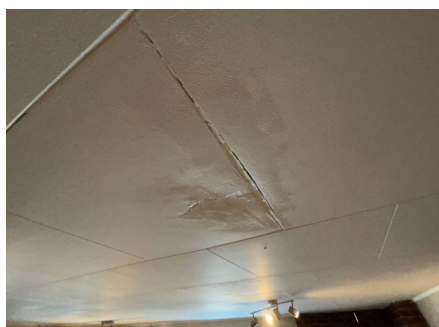
Skade i himling stue.
