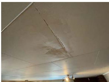
Skade i himling stue.
