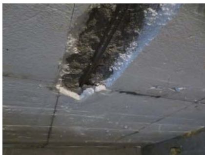
Skade i himling.
