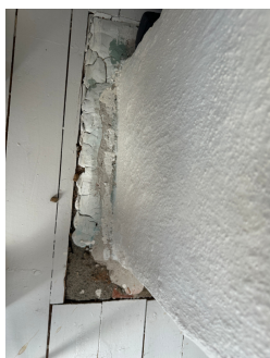
Manglende ildfast plate under feieluke
