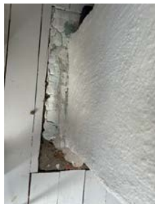
Manglende ildfast plate under feieluke
