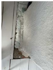
Manglende ildfast plate under feieluke
