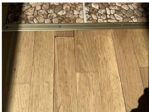
Enkelte gliper/sprekker i parkett TG 2.
