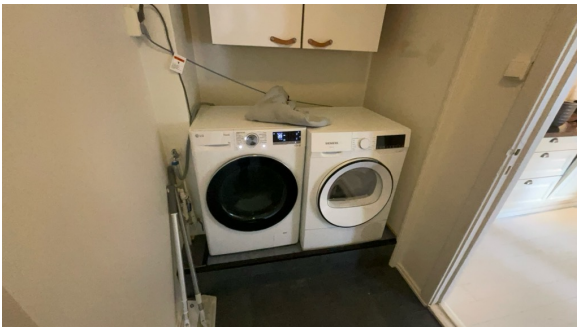
Opplegg for vaskemaskin.
