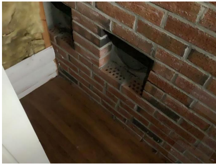
Manglende ubrennbar plate under sotluke.
