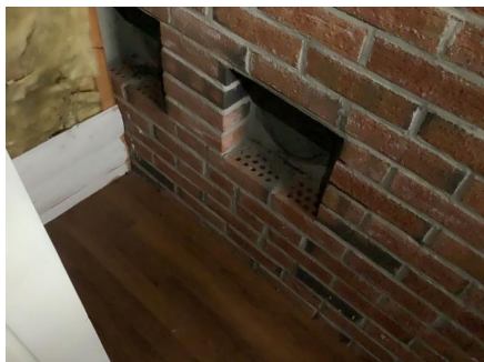
Manglende ubrennbar plate under sotluke.
