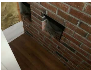
Manglende ubrennbar plate under sotluke.
