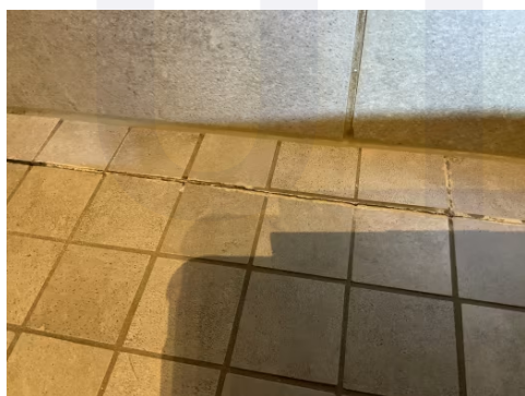
Sprekker i fuger.
