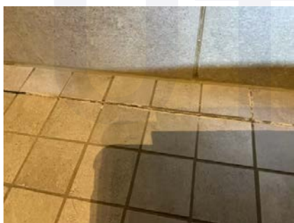
Sprekker i fuger.
