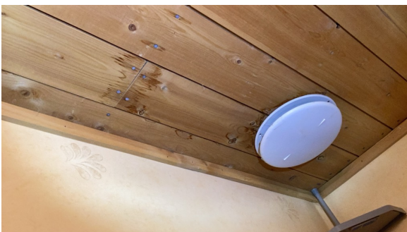
Fuktmerker i himling.
