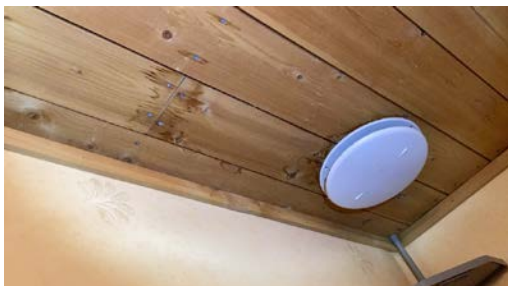
Fuktmerker i himling.
