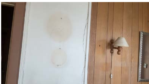
Sprekker i pipe.
