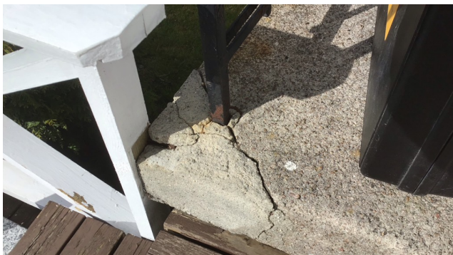
Sprekker i betong trapp
