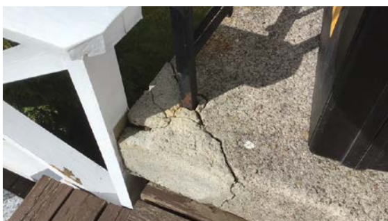
Sprekker i betong trapp
