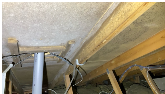
Noe mugg i undertak
