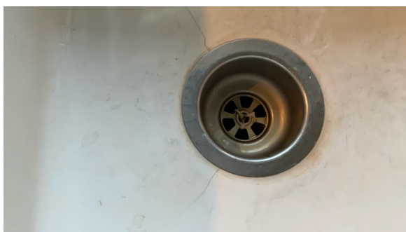
Krakelering i vask.
