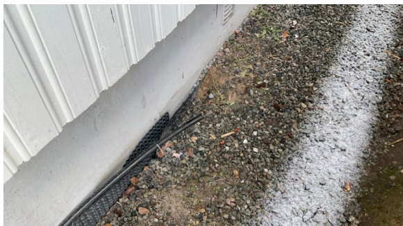
Noe manglende topplist.
